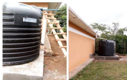
Some of the received and installed water tanks at La Mennais Secondary School
